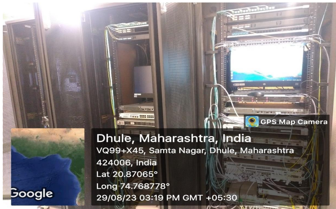
Fig. 15 Maintained Server Room Facilities
