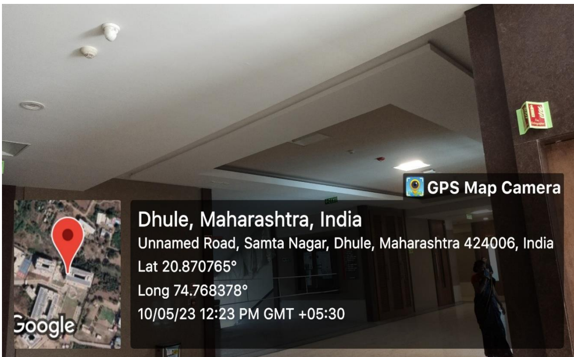
Fig. 14 Maintained Pre Detection Sensor Facilities
