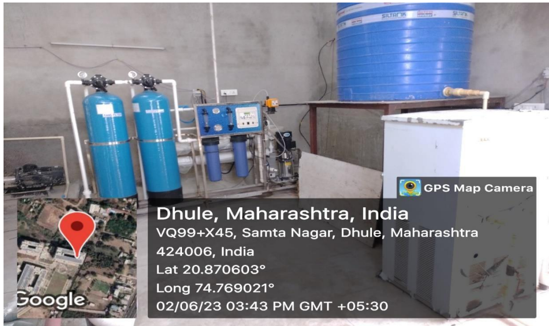
Fig. 8 Cleaned RO- Plant
