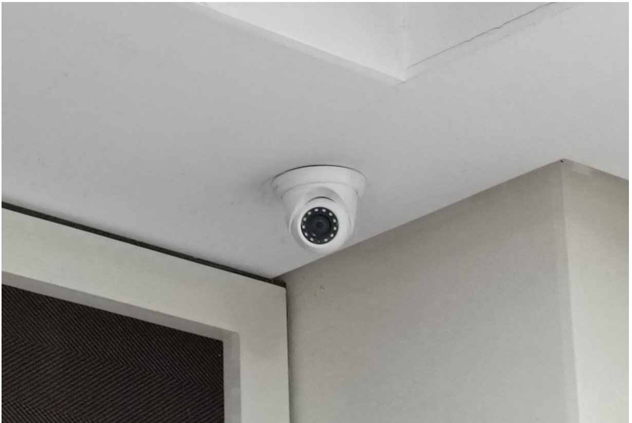
Fig 23: CCTV in each classroom
